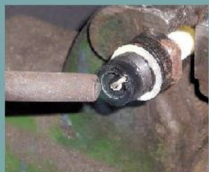
Insulator Heating Up
